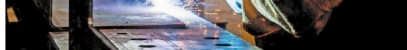
A worker welds a plate to a steel beam at fabricator Walters Group in Hamilton in July. CARLOS OSORIO/REUTERS
